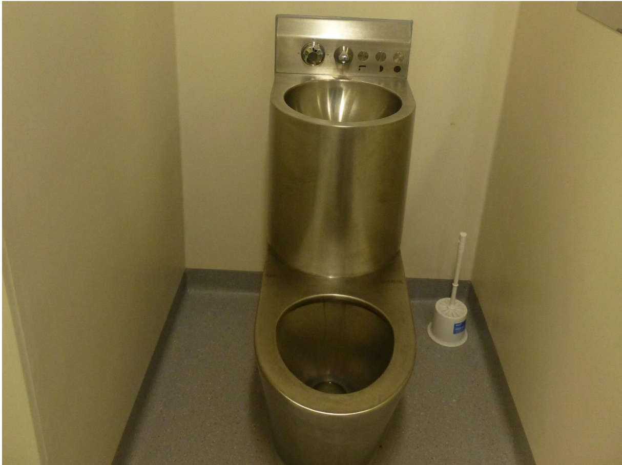
Combined toilet and sink unit, Cassowary compound, YHIDC
