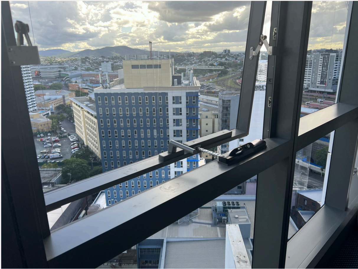
Window opened to maximum extent at Brisbane APOD.
