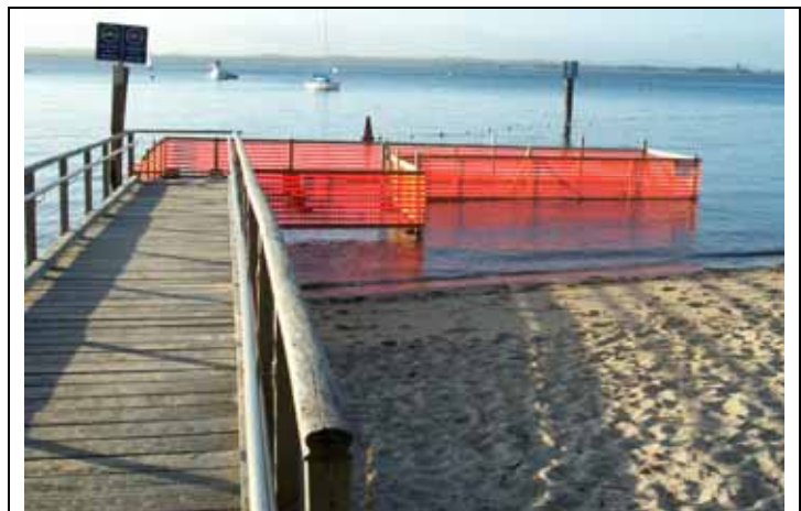
Reconstruction work has commenced on the Little Beach Disabled Access Wharf with an official opening expected in September 2006
